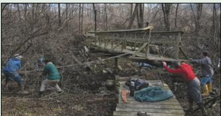
West Jersey crew members started 2012 off by restoring the Appalachian Trail bridge over the Wawayanda Creek.
